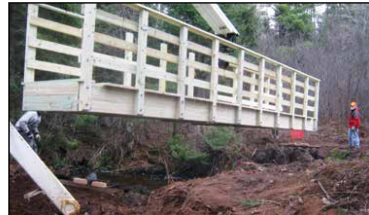
Workers place a bridge above a low area in the diverse terrain characterizing the Agonikak.
