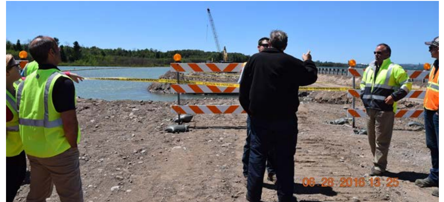
Bridge construction on St. Mary's Rapids with SPAC group tour. The bridge pad is behind safety sign. A portion of the old causeway on the right will be removed.
