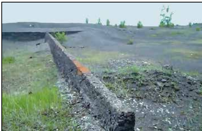
Old retaining wall amid the stamp sands surrounding Gay's abandoned Mohawk Stamp Mill. The sands have degraded a wide beach and benthic zone.
