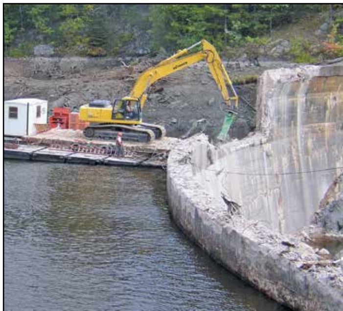
An excavator-mounted jack hammer removes the top portion of the Sturgeon River Dam in the first stage of drawing down the impoundment.
